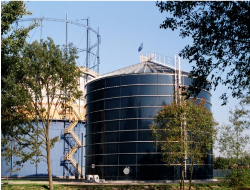
Figure 12: Biogas storage facility at the Wastewater Treatment Plant in Łódź.
